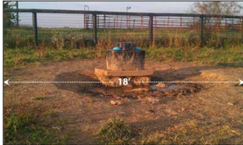
Figure 3-2. Without an all-weather surface, the heavy use area has eroded to the point where the watering facility is almost inaccessible and is no longer frost-proof. The depression also poses a threat to livestock health because livestock have to stand in mud and excrement to drink. Note the diameter of the bare soil area (18'). Photo by Jeff Lehmkuhler
