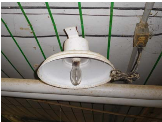
High Pressure Sodium (HPS) light
